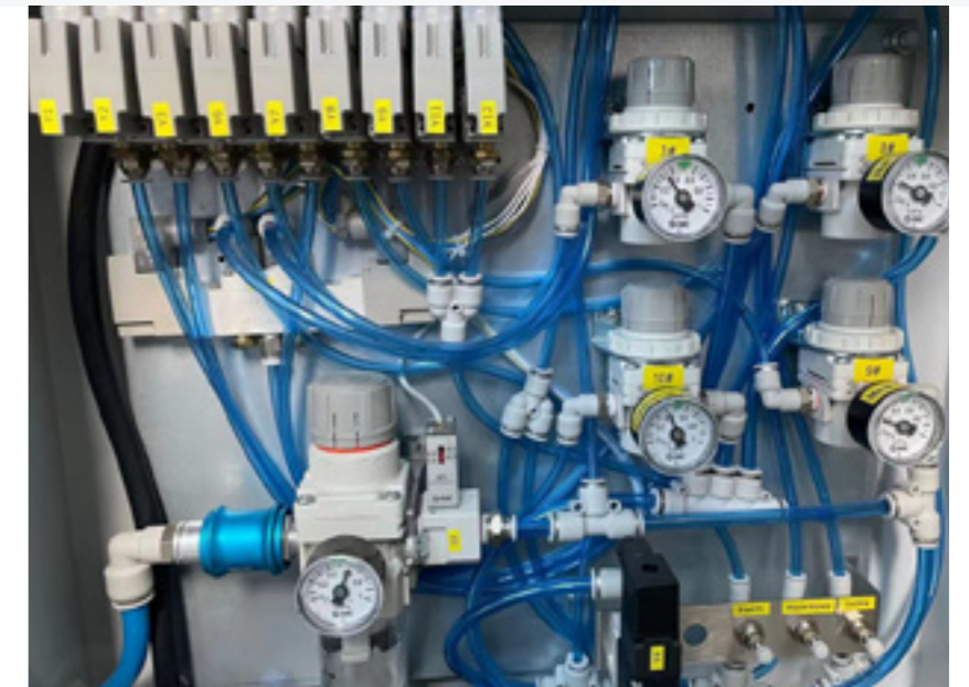
Quality air control part with clean arrangement.
