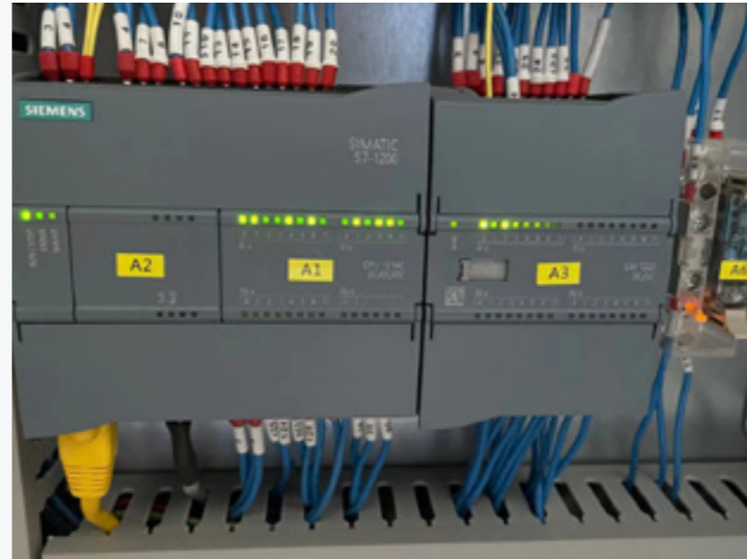
Advanced Siemens PLC
